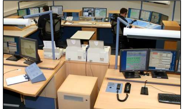
Used in control stations for radio and telephone communication
